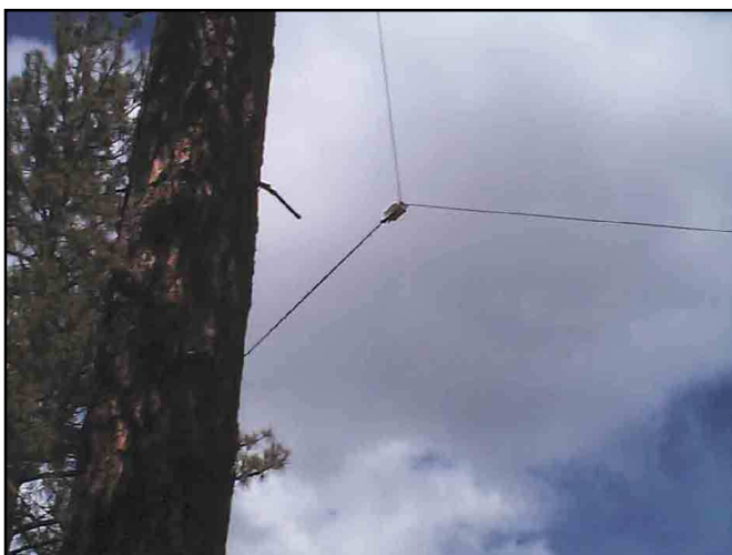
One of the tree supports and insulators. I’m using high-voltage electric fence insulators here. The tie down rope passes through a big screw-eye screwed into the tree.
